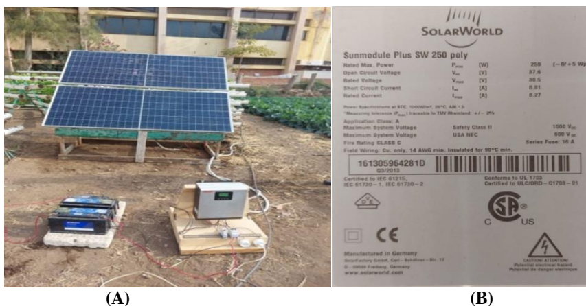
Figure 3. (A-B): A general view of the PV panel system used; (A) the main components of a PV panel system (PV panel, inverter, solar batteries, DC and AC wiring, safety switches, and circuit breakers that are installed between the inverter, batteries, and load), (B) characteristics of the PV panels used.
